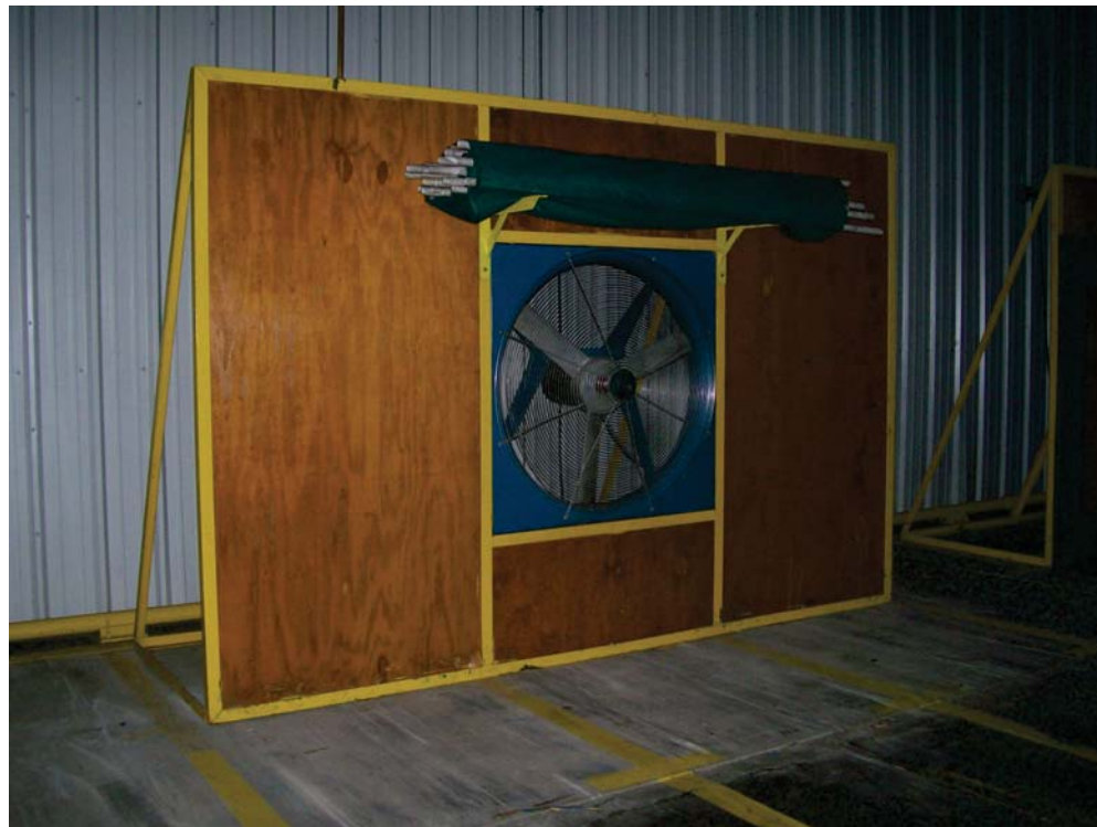
Pre-Cooler in Cold Room
