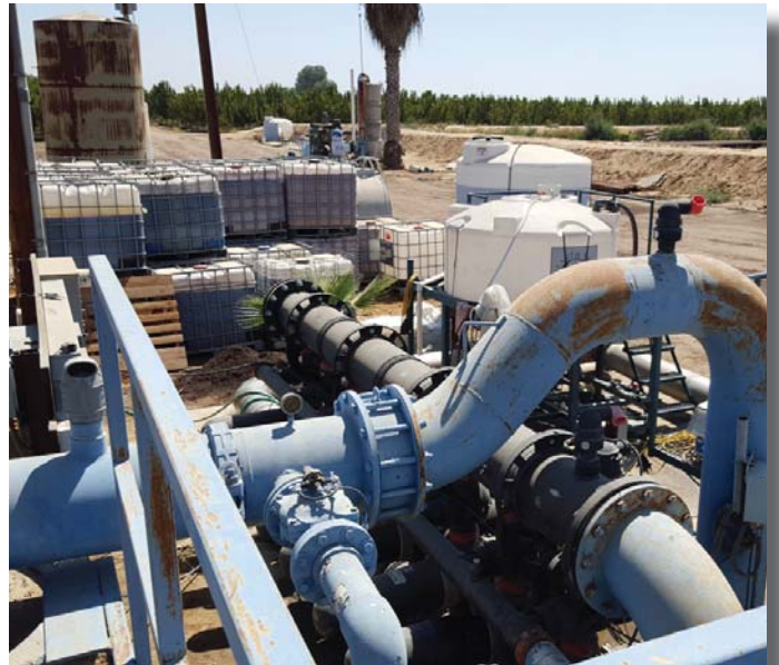
Mix Filter Station
