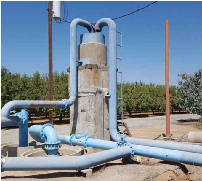
Pump, Well & Outlet
